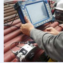
Corrosion Inspection of Boiler Water Wall
